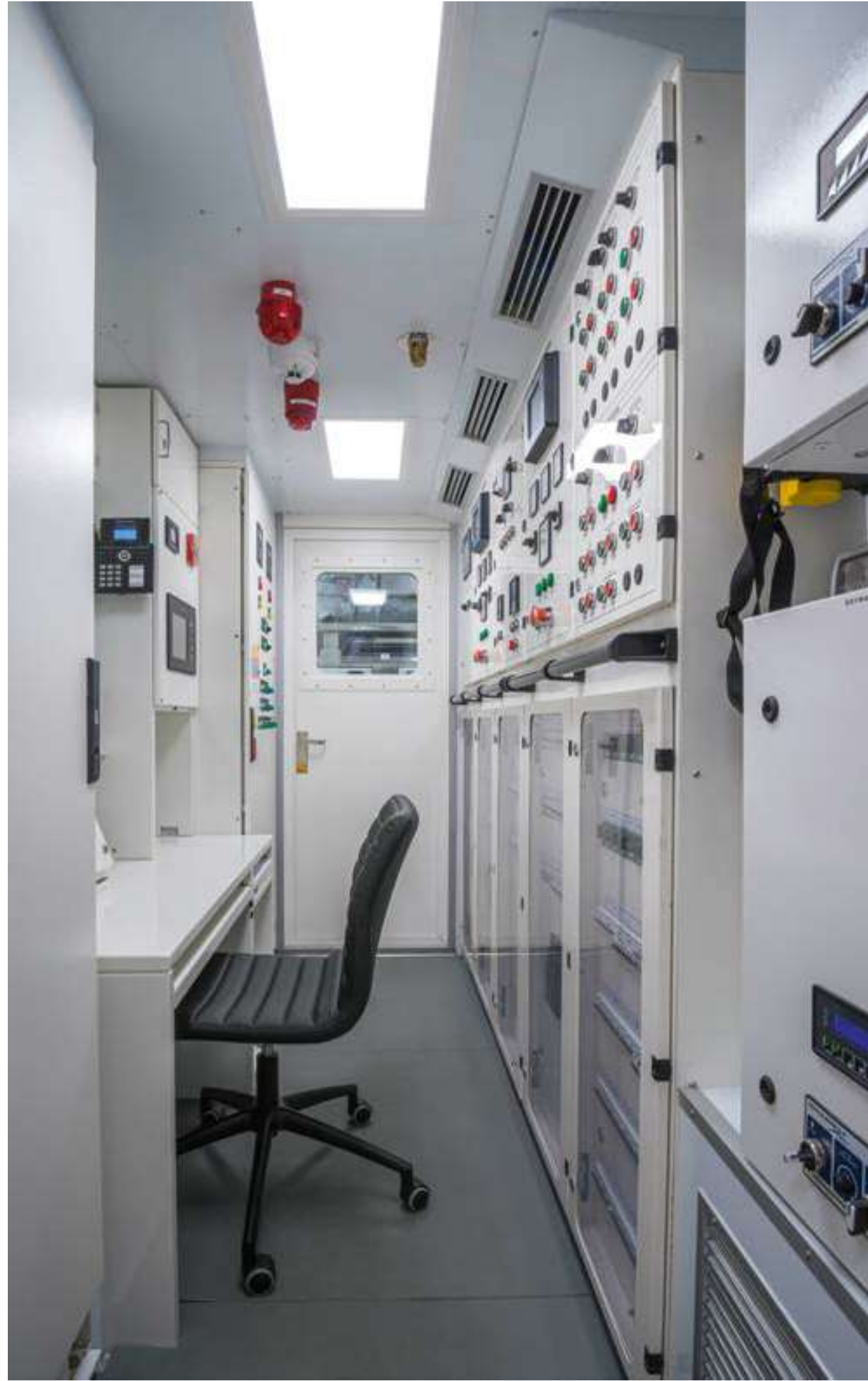
LOWER DECK | ENGINE ROOM
